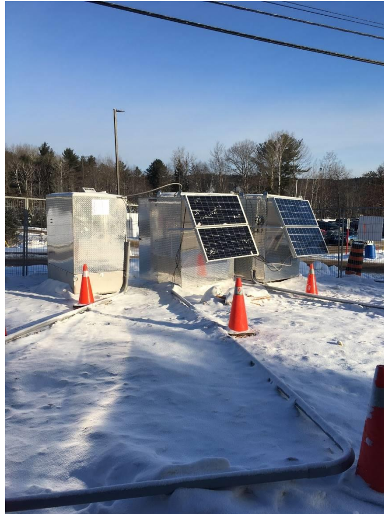
Solar powered tail end odorizer, flowmeter and OdorTracker
