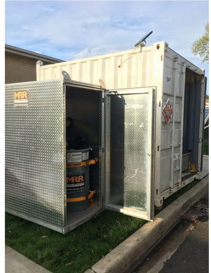
Secured injection equipment
