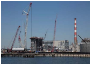
PSEG Power Bridgeport Harbor Station 5 Bridgeport, CT 485 MWs Expected online, June 2019
