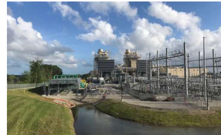
CPV Towantic Energy Center Oxford, CT 805 MWs Online June 2018
